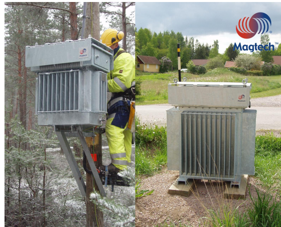
Voltage stabilization MVB mounted on a pole
